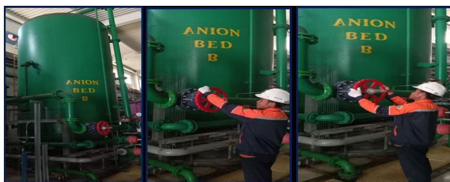
Figure 4. Anion Bed Water Treatment Plant
